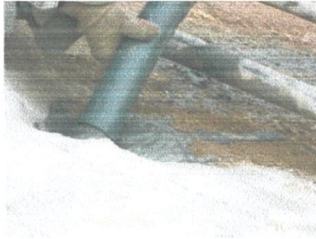
Figure 3.13 Grouted cement came out from the drilled hole.(Draw-off tower)
