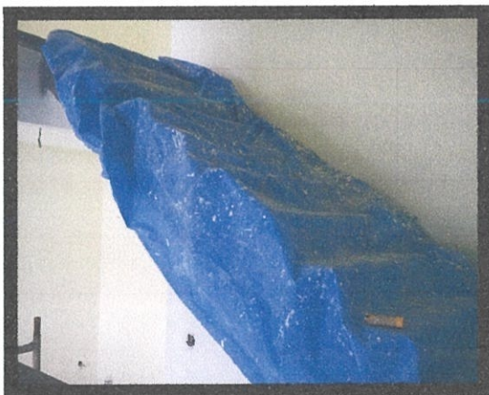
Photo 3.30: The stair was covered with plastic sheet
