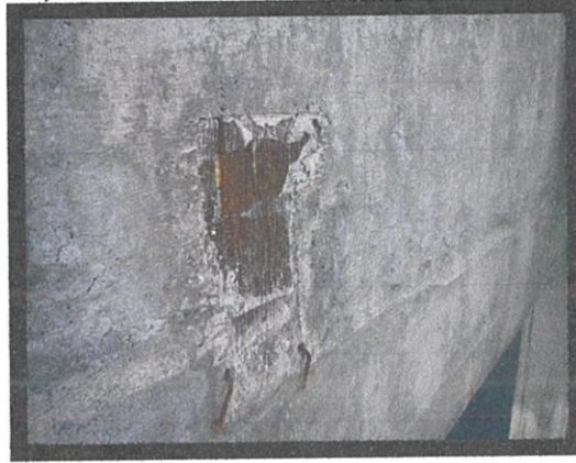
Photo 3.34: The crack was plastered with mortars
