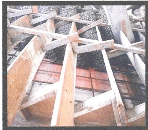
Photo 3.21: The concrete flew in the forms
