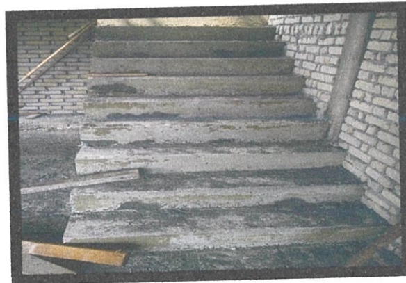
Photo 3.33: The crack was plastered with mortars
