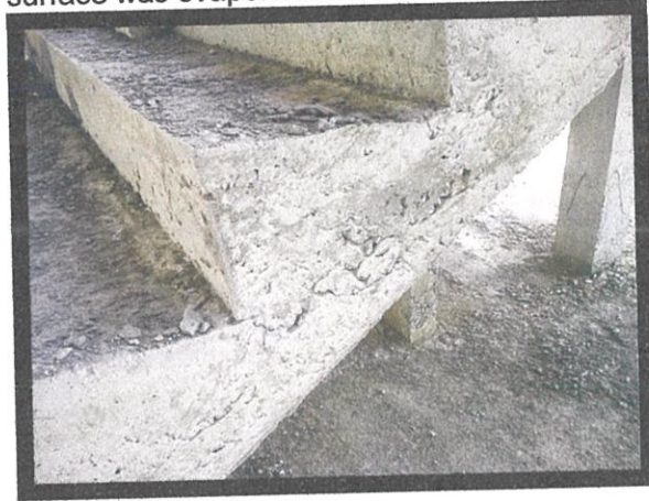
Photo 3.32: The crack on the stair surface
