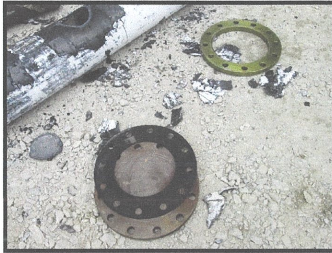
Photo 3.11 Blink flange, gasket and flange
