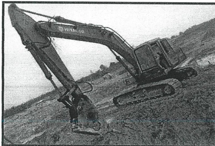
Gambar Foto 4.6 :Breaker
