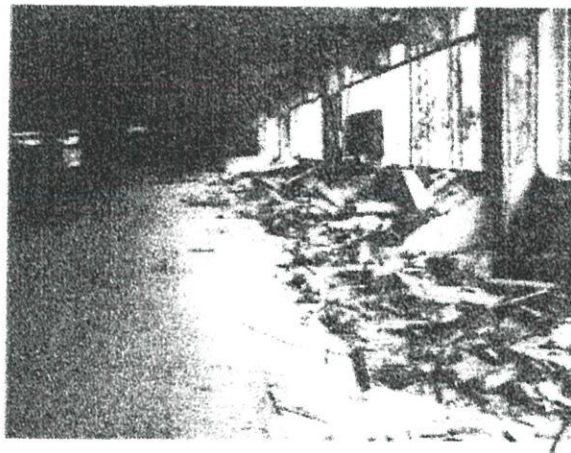
Gambar foto 4.4: Peruntuhan bahagian facade
