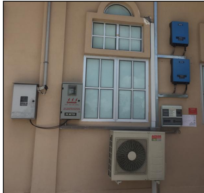
Figure 6: PV system indicator on Ar-Rahmaniah Mosque
