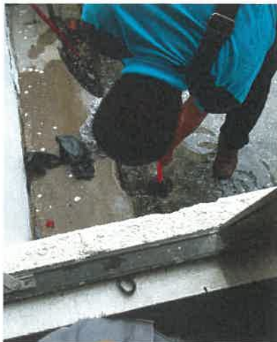
Clogged pipe and drainage
