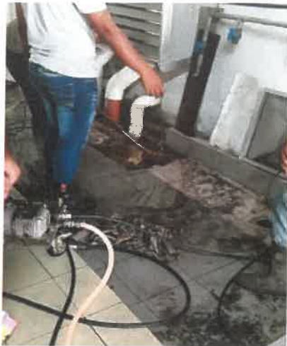
Clogged Sewage tank
