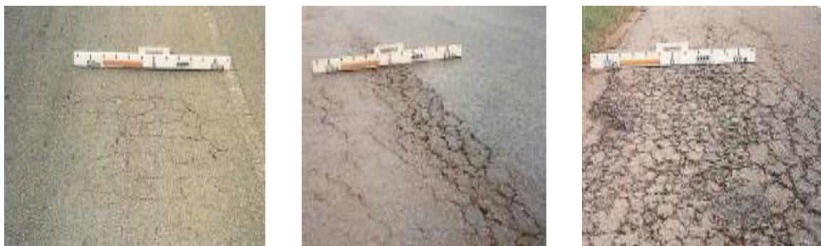
Figure 1. Classification of crack's severity from low, moderate to high (left to right) [7]
