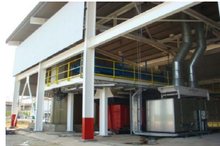
Picture 1. A typical installation of a Sludge Drying Plant on an Oil and Gas Processing Plant.
