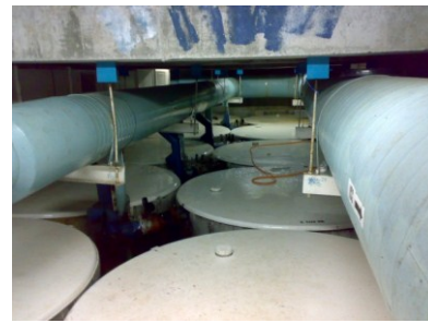
Figure. 4 Ice storage tank at the indoor (Underground)
