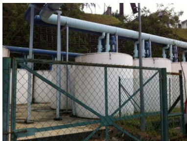
Figure. 3 Ice storage tank at the outdoor (Parking lot)
