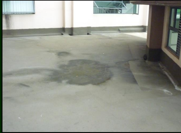
Figure 6.9: Waterproofing failure at Block B7
