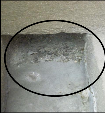
Figure 6.8 :The Blistering of Waterproofing Cause By Weather Expose.
