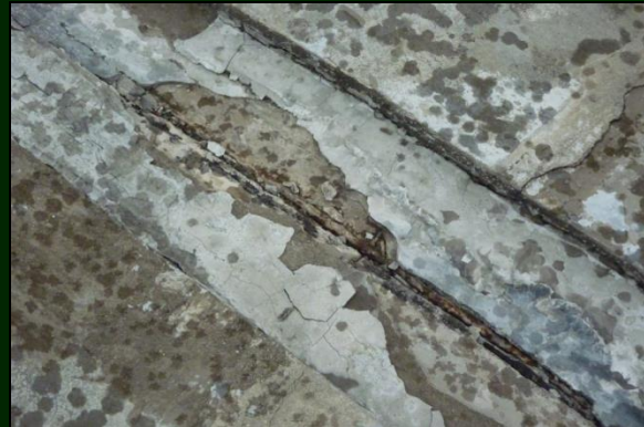
Figure 6.3: Surface crack of cementitious waterproofing system at the roof top of Wisma Putra 1 due to weather expose.
