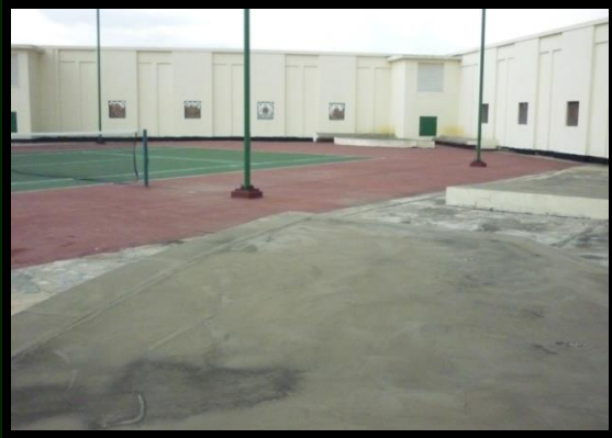
Figure 6.1: The waterproofing failure at roof top of multipurpose hall Wisma Putra 2
