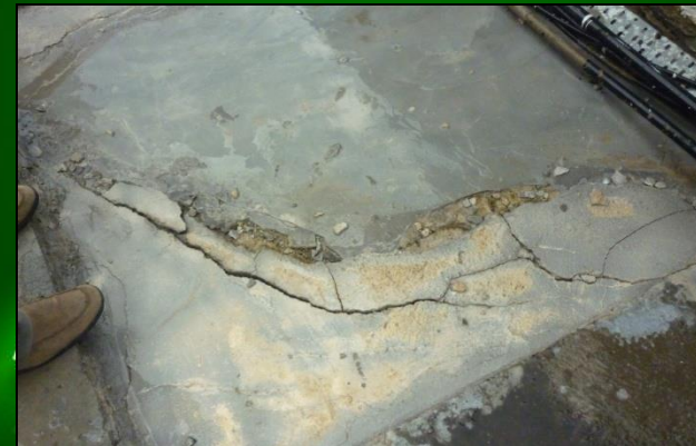
Figure 6.4: Splitting of cementitious waterproofing due to weather expose and poor workmanship.
