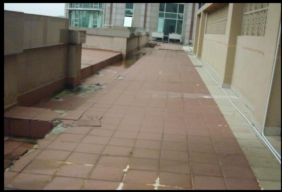
Figure 6.5 : Waterproofing Failure at Atrium because of Deterioration
