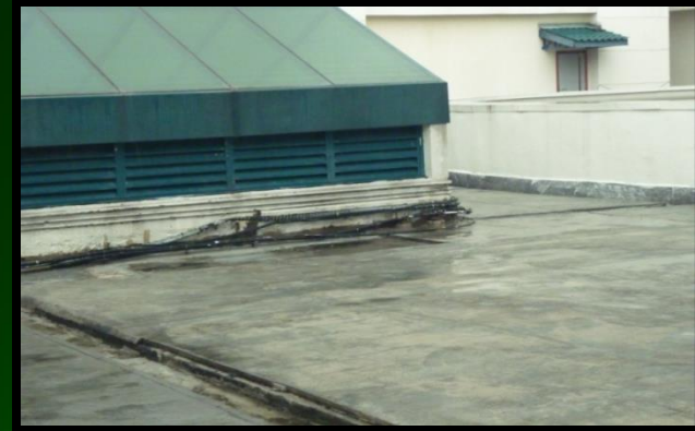
Figure 6.2: The Waterproofing Failure because of Repairing Work
