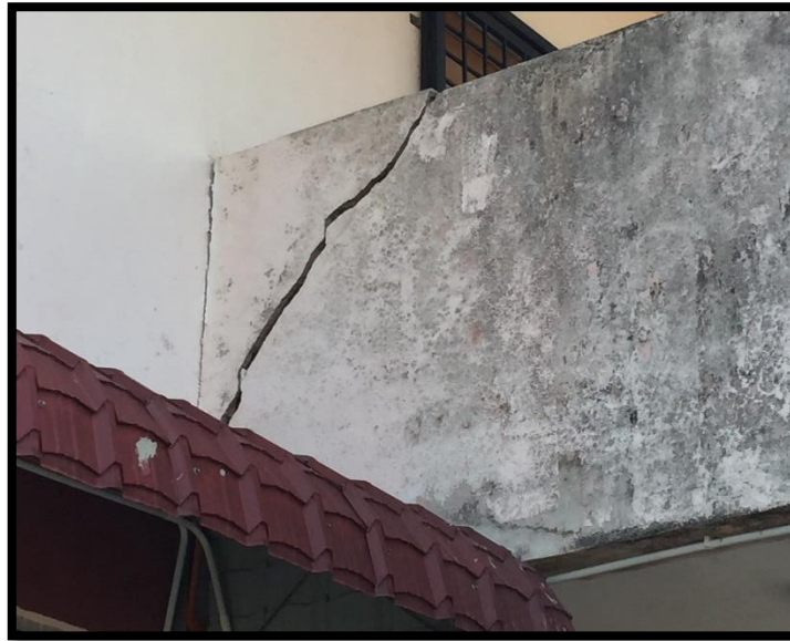
Figure 3.4: the concrete crack on parapet wall
