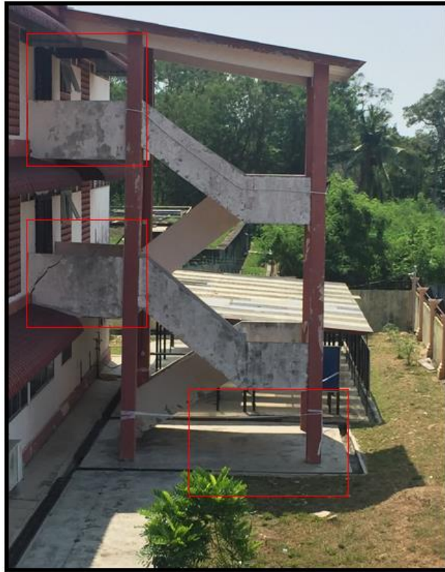
Figure 3.19: the area that appear the defect on staircase.
