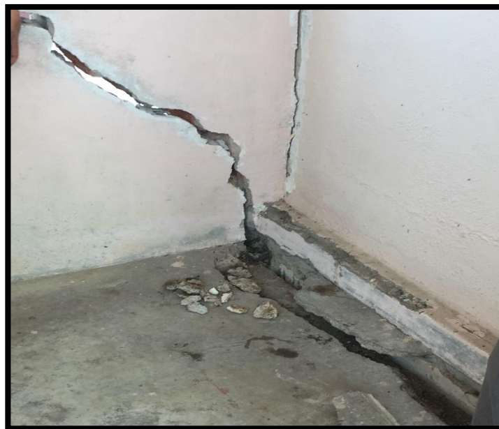
Figure 3.5: the crack on the slab of additional staircase
