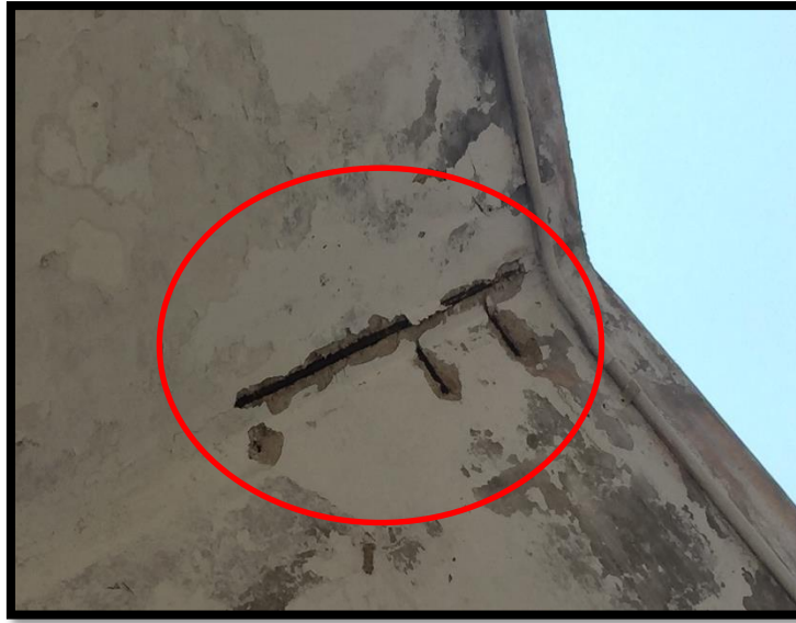
Figure 3.6: the concrete spalling and concrete delamination
