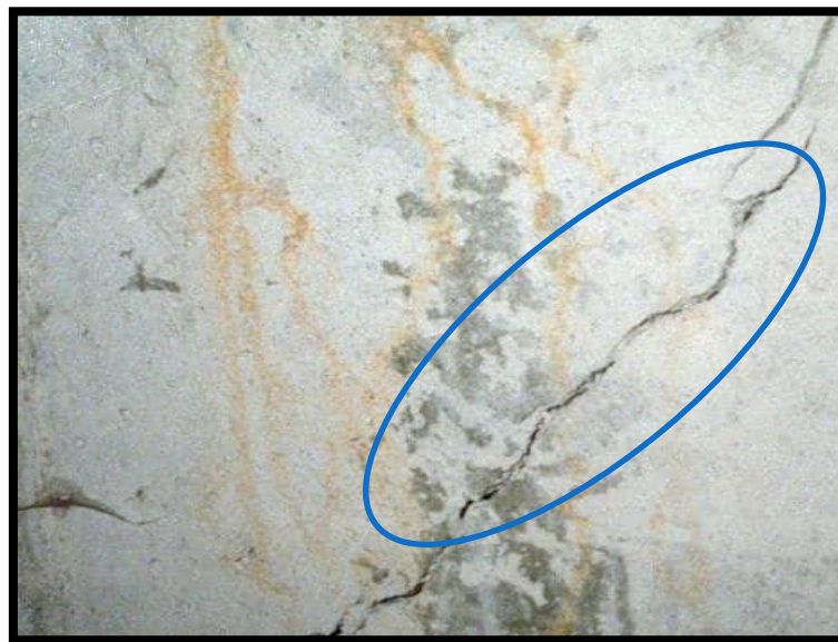
Figure 2.11: The example of diagonal crack
