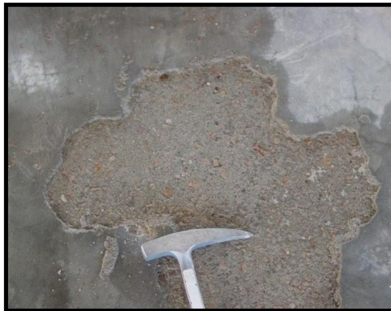
Figure 2.15: the example of delamination
