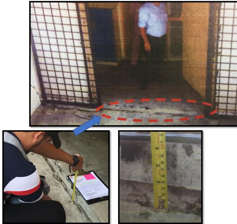
Figure 3.23: crack on diagonal parapet wall.
