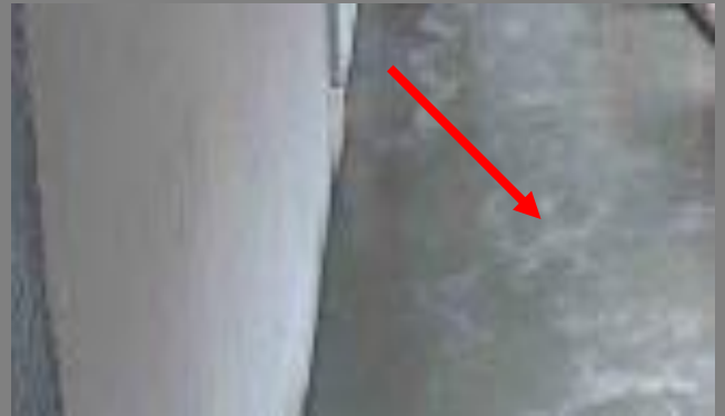
Figure 3.4 Floor Was Be Cement Render
