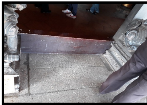
Photo 3: The high sill that prevented the wheelchair to get to the other side of the building.
