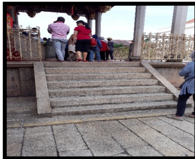
Photo 1: There are no facilities such as ramps and a hand holder provided for senior citizens and disabled people to visit the heritage building.
