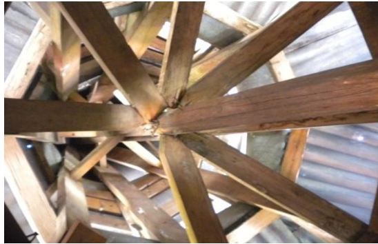
Fig. 6. Macu pillar located on the second floor, its length reaches the fourth floor of surau. Sources: Personal Documentation.
