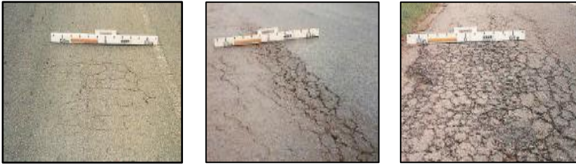
Figure 1: Classification of crack's severity from low, moderate to high (left to right).
