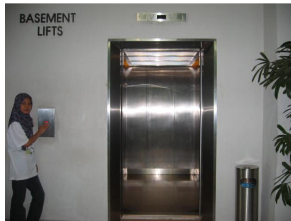
Figure 7: Basement lift at MRCB, Shah Alam
