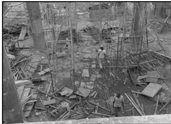
Picture 1: Shown that workers did not wearing safety helmet. Site visit to Air Itam Mosque Project dated 19 Ogos 2008. (JKR Project)
