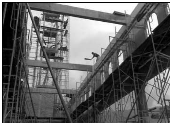
Picture .2: Shown that wokers did not wearing safety helmet and safety belt. Site visit to Air Itam Mosque Project dated 19 Ogos 2008. (JKR Project)
