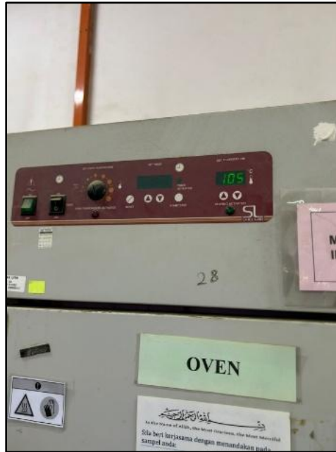
Figure 3.7 Temperature Setting of Oven
