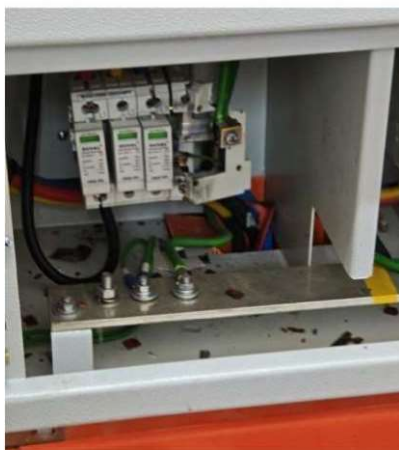
Figure 1: Faulty SPD Observed in Electrical Panel Due to Surge Impact
