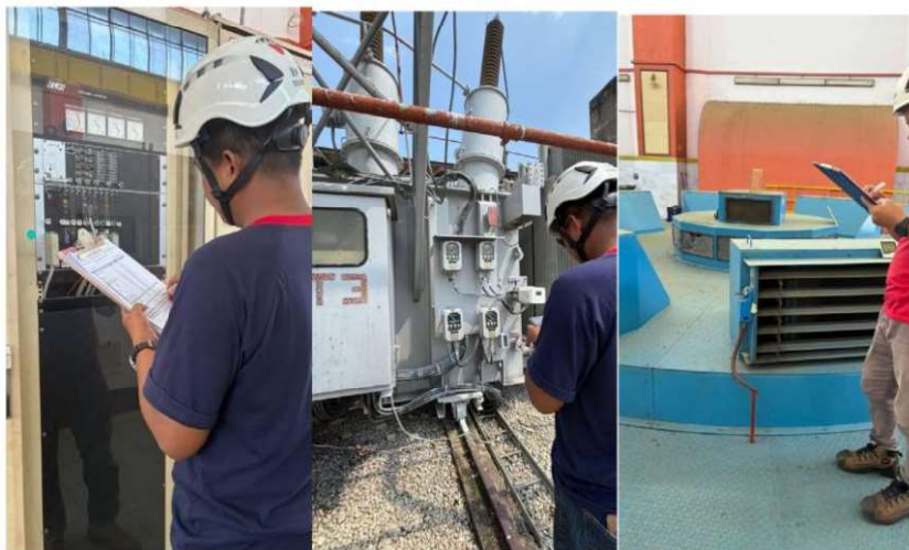
Figure 1: Observing System Operations and Monitoring Electrical Parameters
