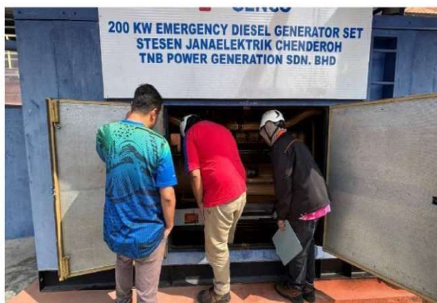
Figure 4: Emergency Diesel Generator Inspection
