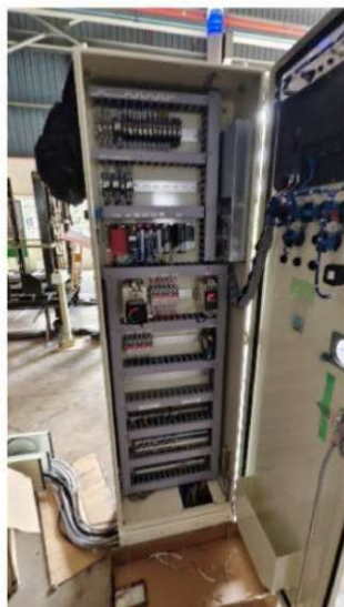
Figure 2: Inside of Mitsubishi PLC
