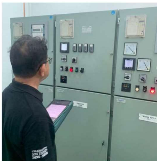
Figure 1: Monitoring Electrical Switchgear Control Panels Using Digital Metering Devices to Evaluate Power Distribution System Performance
