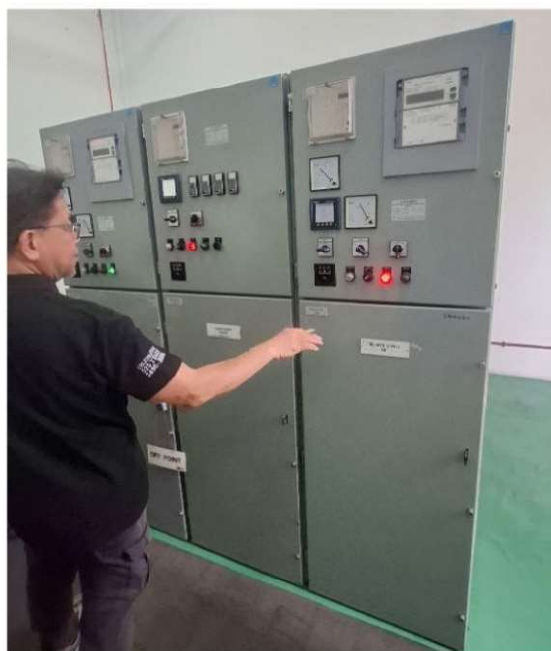
Figure 2: Learning the Operation and Monitoring of High-Voltage (HV) Switchgear Panels Under Professional Supervision
