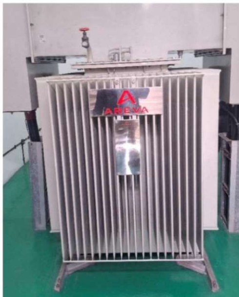
Figure 1: Close-Up View of the AREVA Backup Transformer, A Critical Component for Power Reliability
