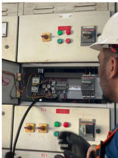
Figure 1: Electrical Control Panel During Inspection and Troubleshooting
