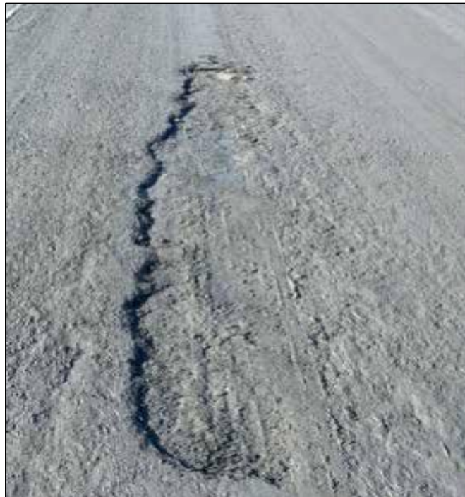
Figure 3-15 The Surface Must Not Be Slurries, Since This May Result in Delamination and the Formation of a Soft Crust.
