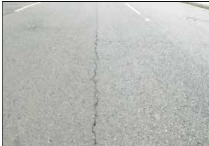
Figure 3-13 Longitudinal Shrinkage Cracks May Appear If 'Full' Compaction Is Applied Near a Longitudinal Run of the Stabiliser Where Multiple Runs Are Used on Site.
