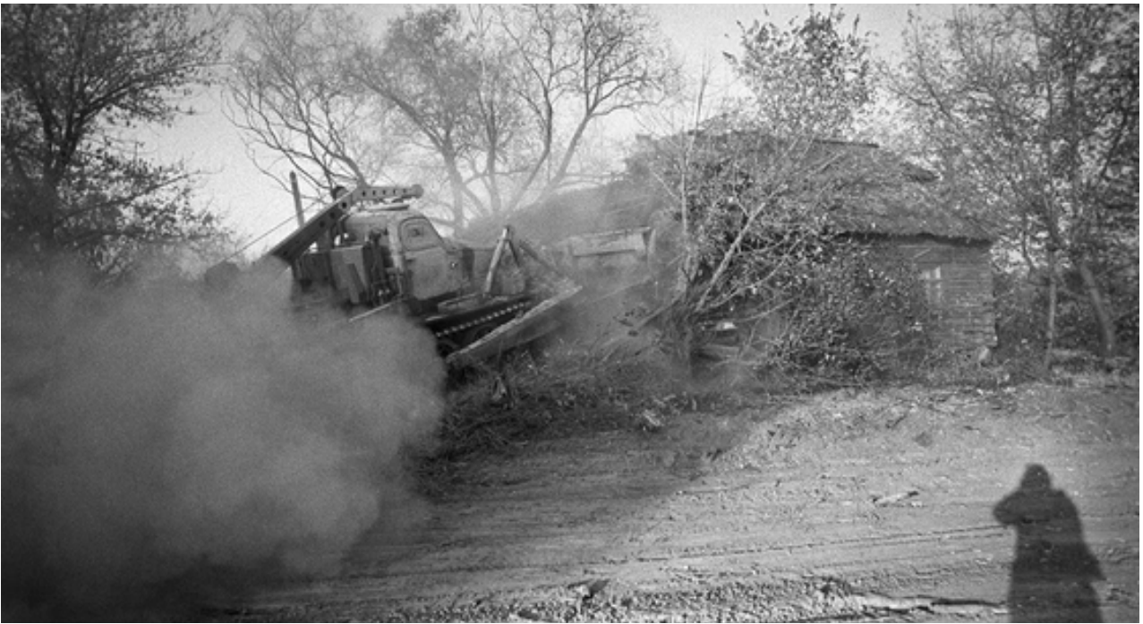
A bulldozer digs a large trench in front of a house before burying the building and covering it with earth. This method was applied to entire villages that were contaminated after the Chernobyl disaster.
