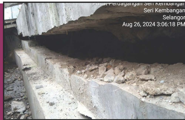
Figure 1 Settlement under the building
