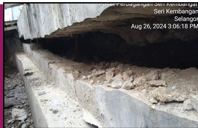
Figure 1 Settlement under the building
