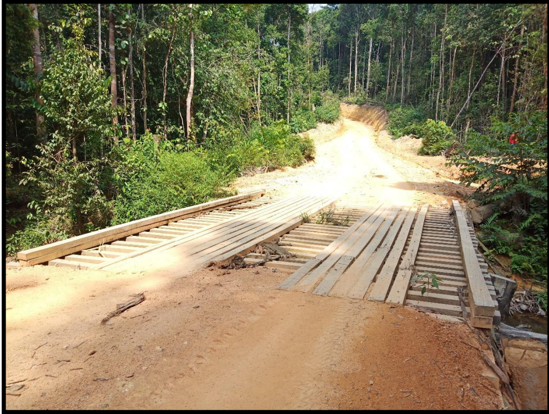
Plate 1.1 Timber Bridge with Log Girder Construction Typical of Temporary Forest Access Infrastructure
