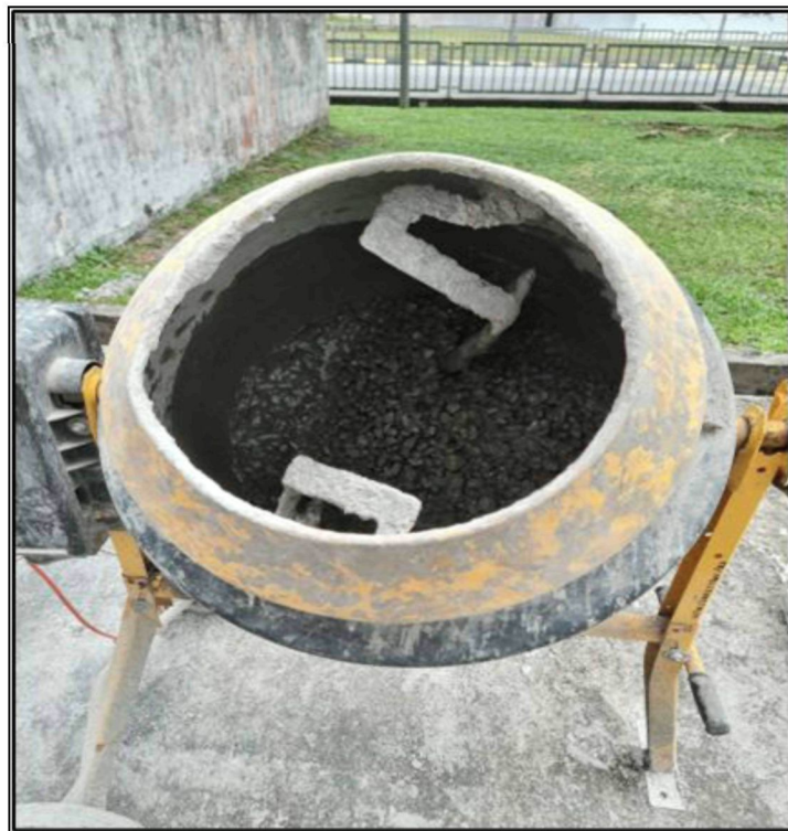
Figure 3.36 The Concrete Ingredients Mixed Within A Concrete Mixer In Batches According To Their Admixture Compositions
