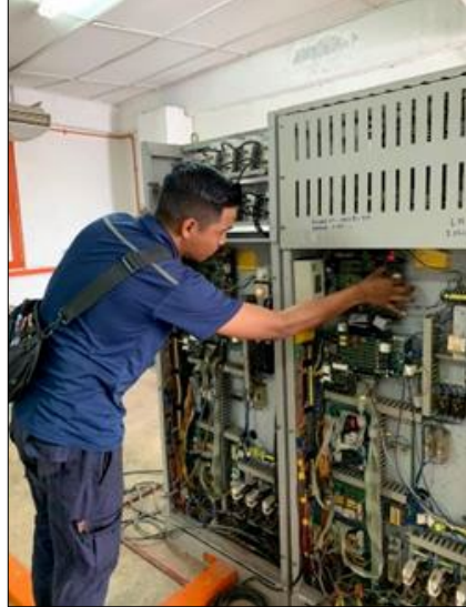
Figure 4: Electrical Control Panel Inspection
