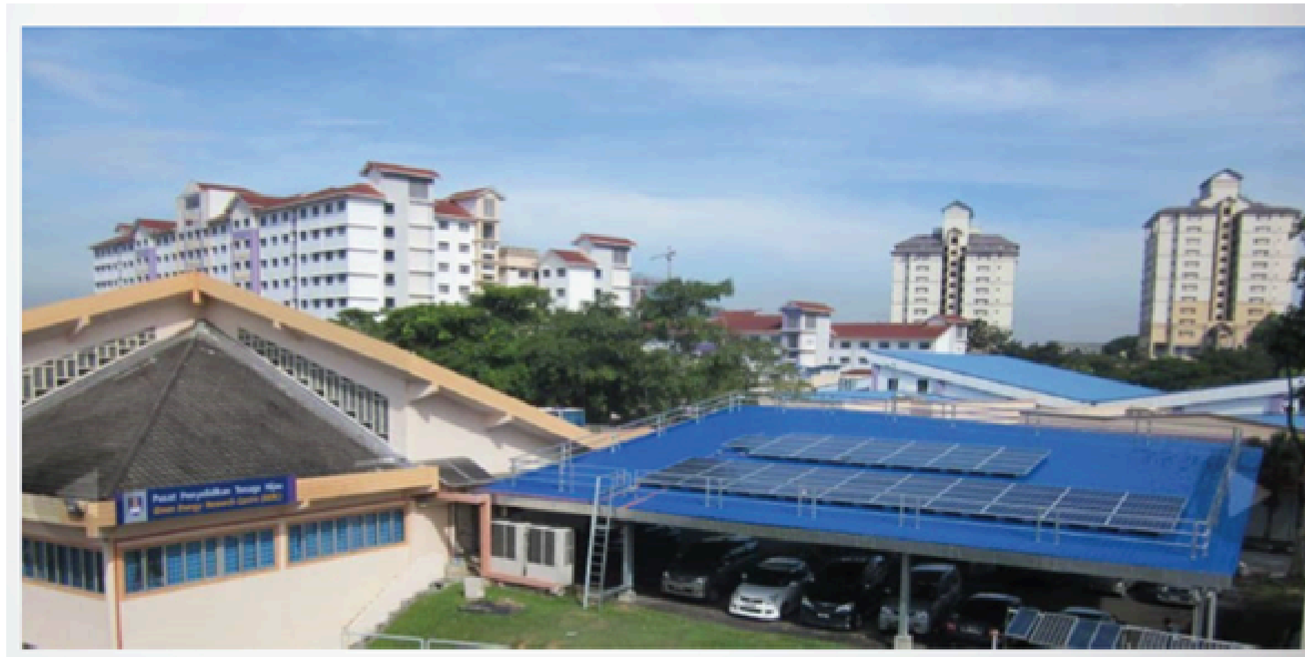
Photovoltaic roof solar panel at particular building with total of 20kW
