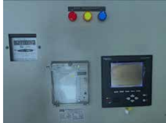
Figure 2.14: Smart Meters Data Loggers and Data Recording
