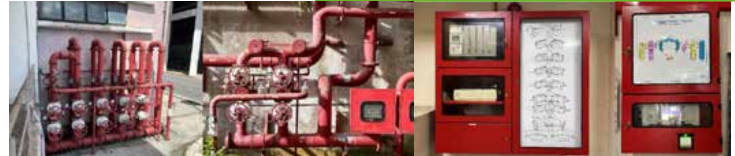
Figure 2.9: Firefighting Facilities and Monitoring Systems
