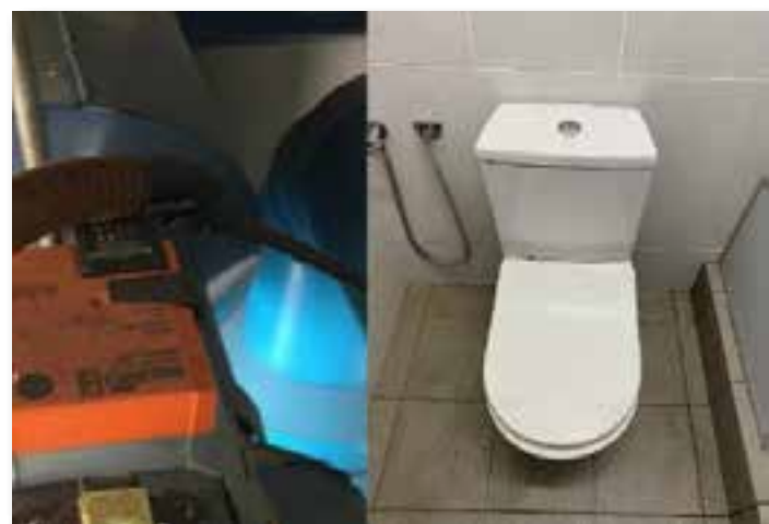
Figure 4.8: Auto Sensor and Dual-flush toilet
