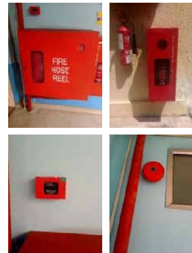
Figure 1.13 (a,b,c,d,e,f): Fire Hose Reel, Fire Extinguisher and Emergency Break Glass Panel
