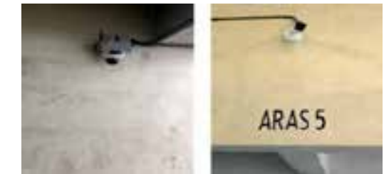
Figure 1.12 (a,b): Closed-Circuit Television (CCTV)
