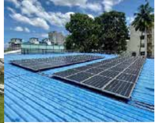
Figure 2.15: 19 kWp Solar PV System (GERC) - Kolej Teratai
