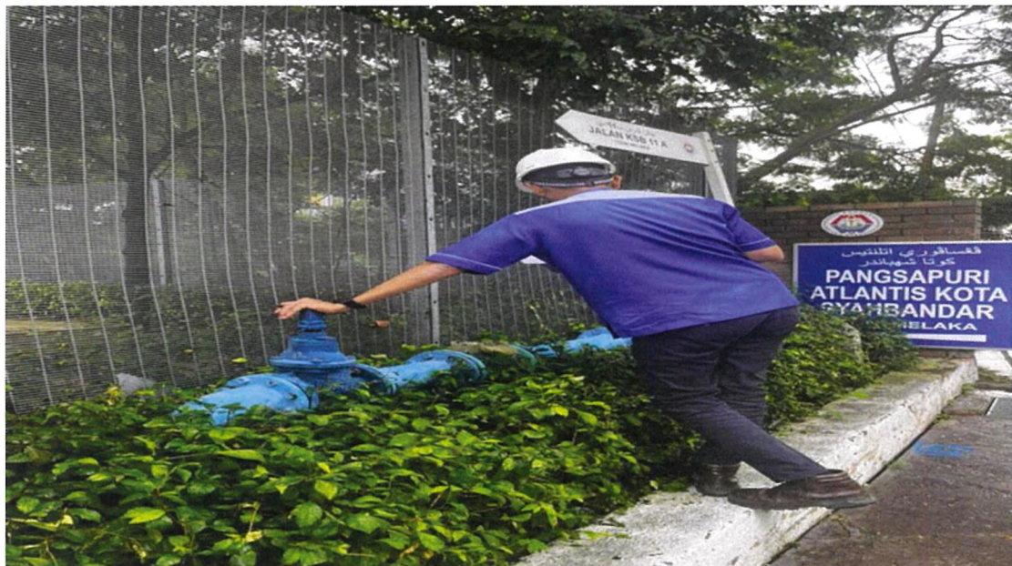
8.6 Monthly Checking on meter at Bandaraya Melaka Area
