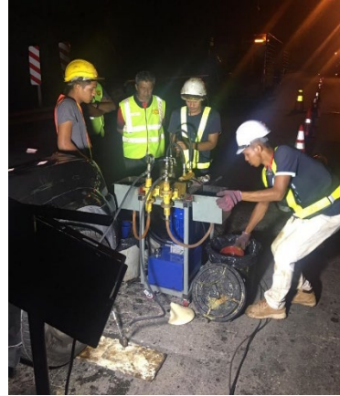
Figure 10. Injecting the PU foam mixture at designated injection pressure in situ into the ground (Zainuddin et. al., 2021).
