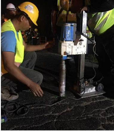
Figure 9. Coring of the asphalt layer before injecting PU foam underneath the piled embankment (Zainuddin et. al., 2021).
