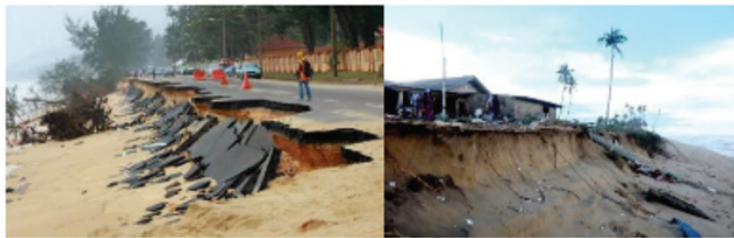
Figure 7. Erosion on (a) Teluk Lipat Dungun, (b) Tok Jembal Kuala Terengganu in December 2011
