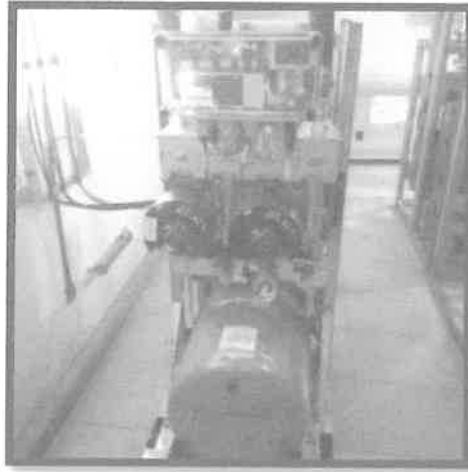
The figure 3.4.1 Air Cooling System for Transmission Room.
