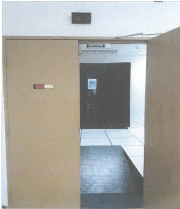
Figure 10: Server room from outside
