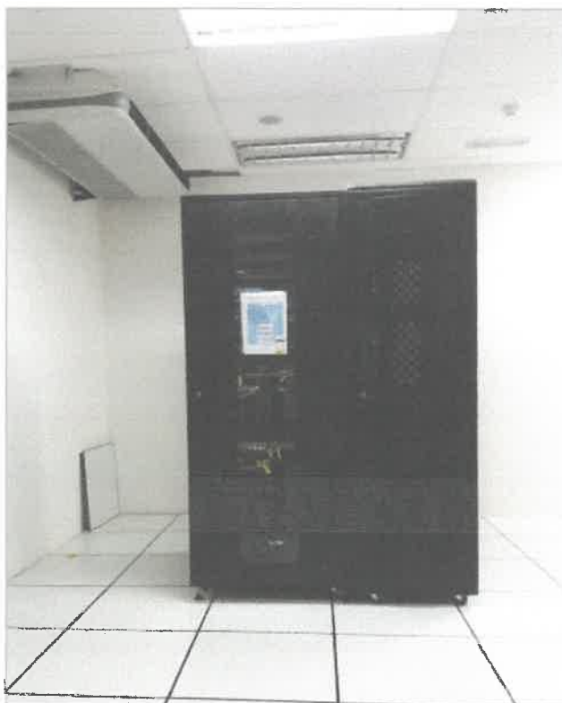
Figure 11: The server in server room
