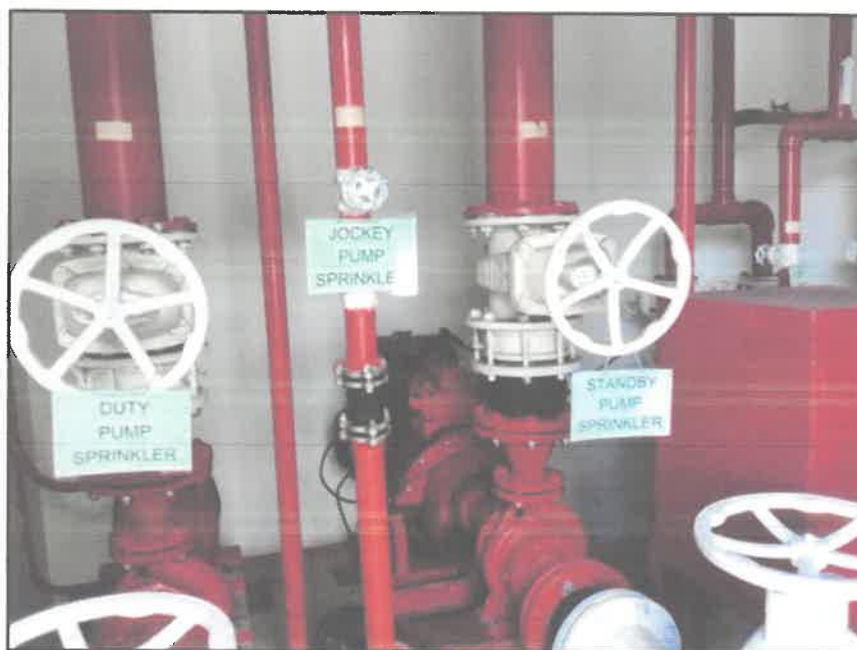
Figure 18: Water sprinkler pump
