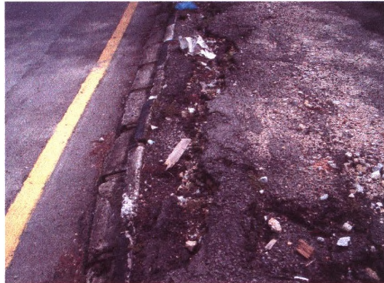
Figure 1.1: Settlement at pedestrian pavement.
