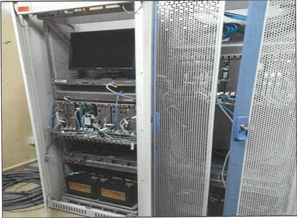
Appendix 48: The wired rack that was connect with 3000 extension wired
