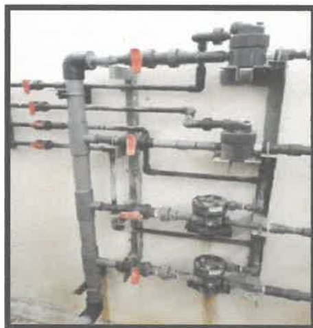
Figure 3.18: Piping of Chlorine
