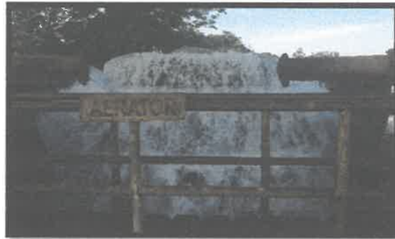
Figure 3.12 : Circular Cascade Aerator
