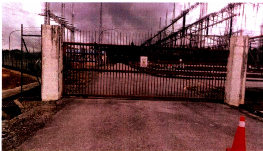
Selangau Sub-Station 245kv
