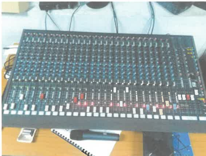
Figure 3.22: P.A system in Dewan Kenanga, MPSP
