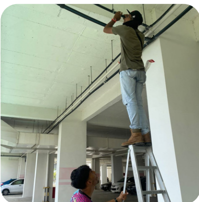
Assist maintenance team on putting up bird fence at car-park lot as report.
