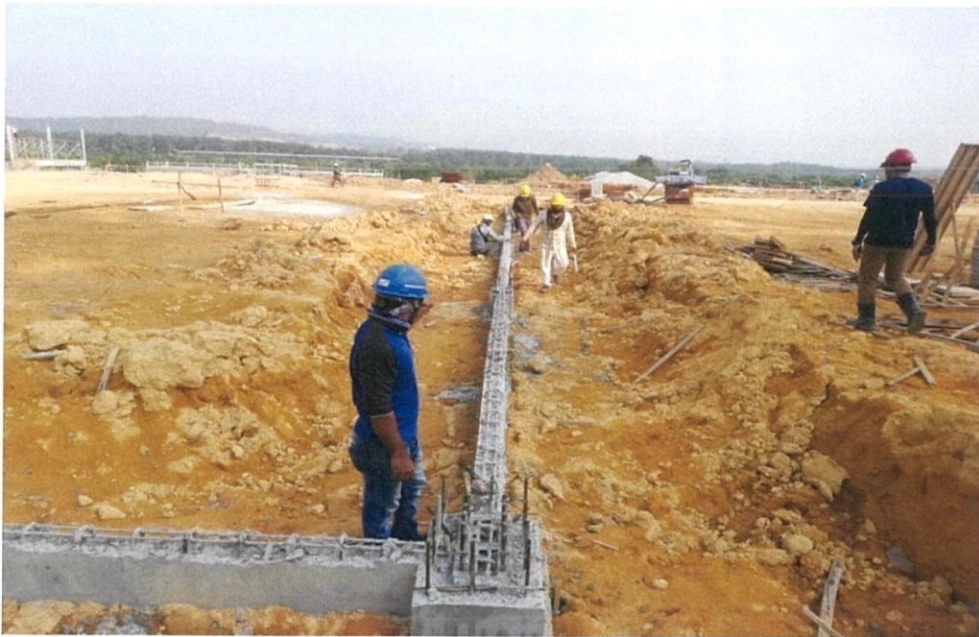
Figure 3.10: J-bolt installed into the form and has been layered with a concrete float
