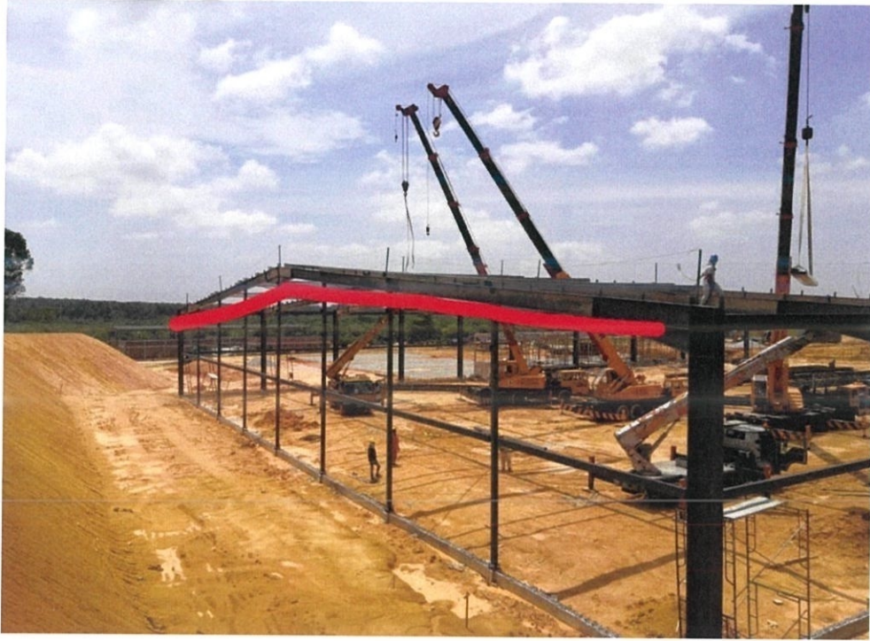
Figure 3.29: Unregulated purlin at lawn bowl
