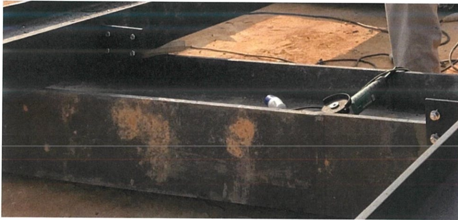
Figure 3.25: Defect and faded colour on steel
