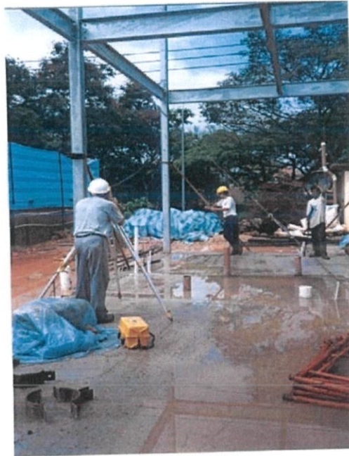
Photo 3.8: Using the total station to check the verticality and temporary bracing were installed.
