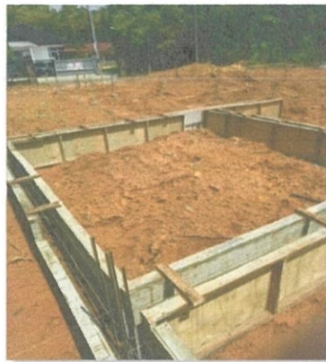
Photo 3.22: The reinforcement were place in the formwork and reinforcement were tied together.
