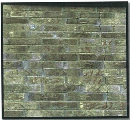
Figure 13 Thermal cracking (Sources: Google)
