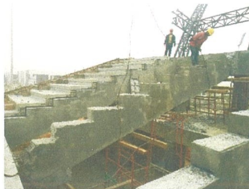
Figure 3.24 Beam should be removed
