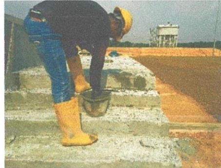
Figure 3.21 Recover the honeycomb defect
